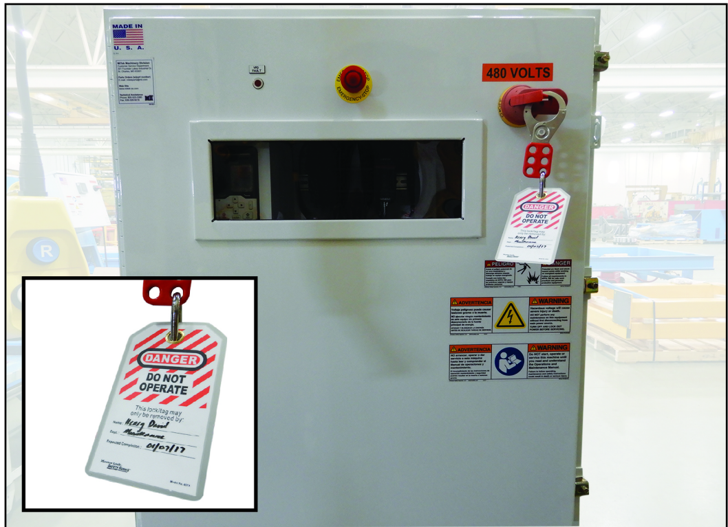
Main electrical enclosure on a RailRider Pro shown above.
